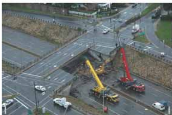
Figure 3.1 Collapsed Portion of the de la Concorde Overpass 1
